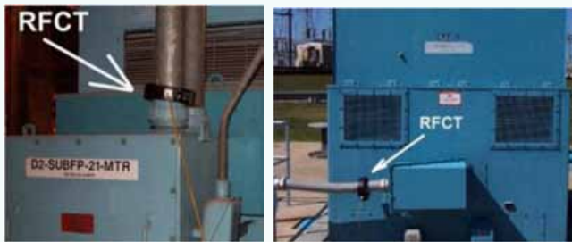
Fig. 1: Placement of RFCT to collect EMI data
